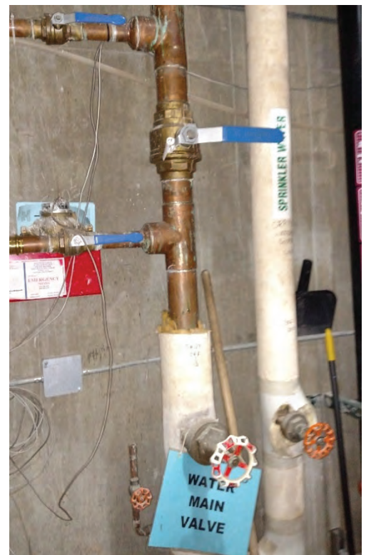
PLMB #2 Main Building & Irrigation Risers
