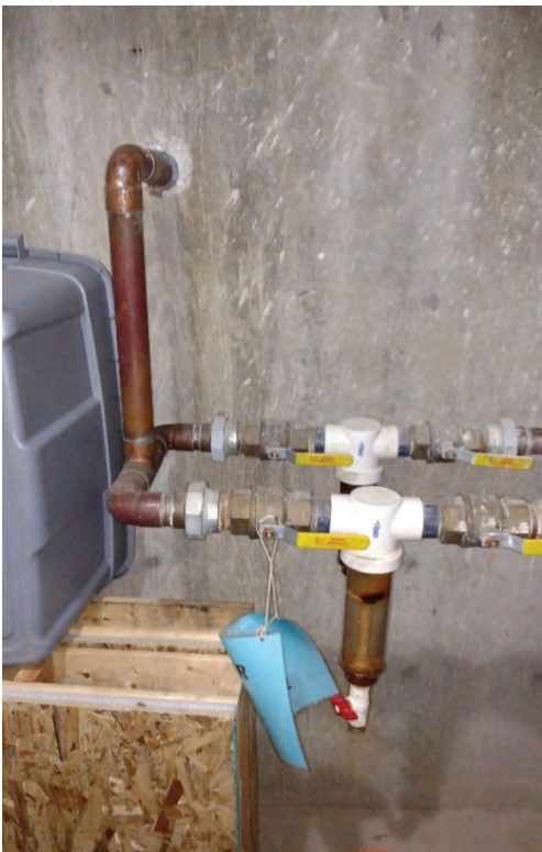
PLMB #1 Existing 2" water service with filters
