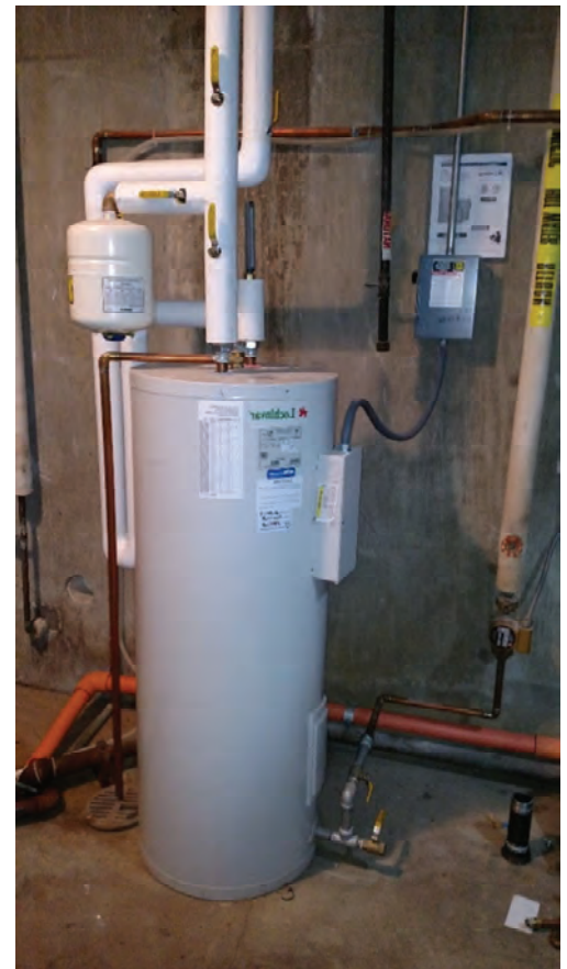
PLMB #4 Electric Water Heater
