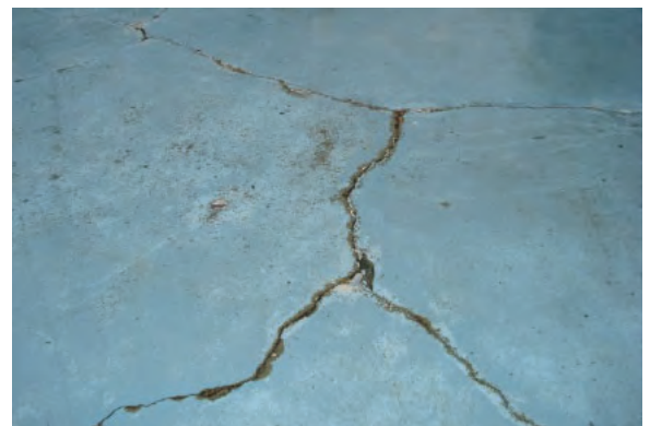
Photo 1: Concrete cracking and vertical displacement
