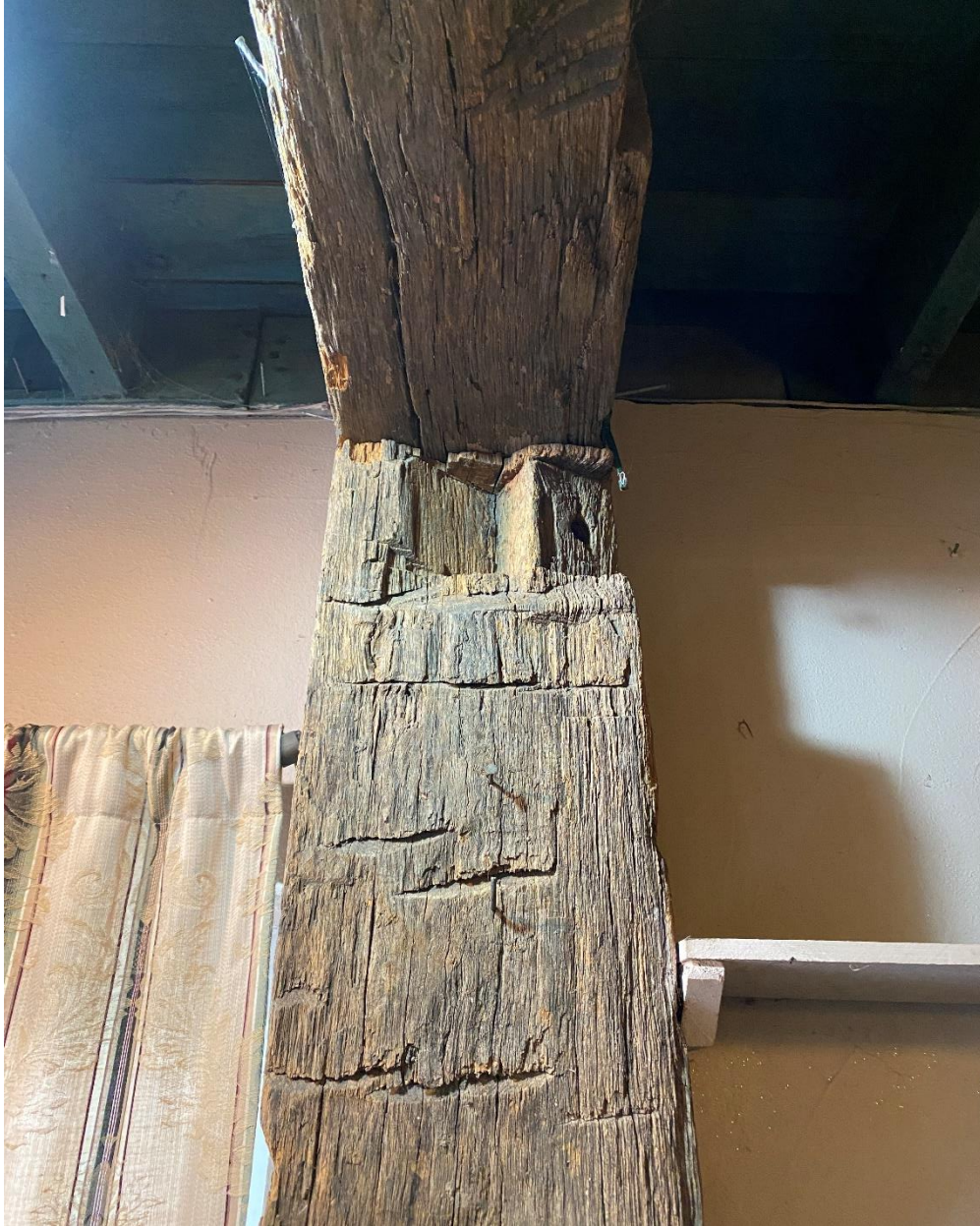
Notch in beam indicates beam was originally used in a different building and used in this building for aesthetic purposes.
