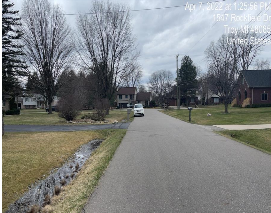
Photograph No. 1: Rockfield Drive- Heading West Date: 04/7/2022 Photographer: Richard Boateng & Genevieve Schneemann
