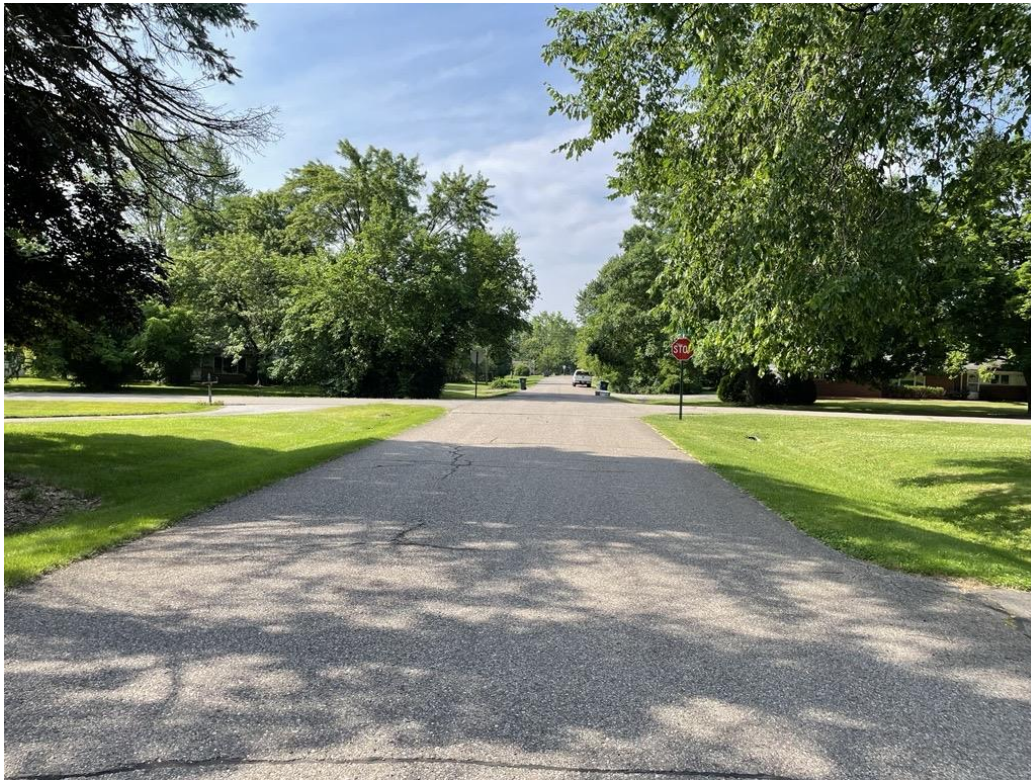
Photograph No. 8: Donaldson Road - Heading South Date: 06/18/2024 Photographer: Lauren Hull
