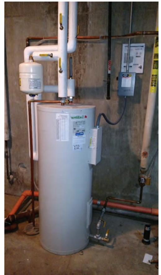
PLMB #4 Electric Water Heater
