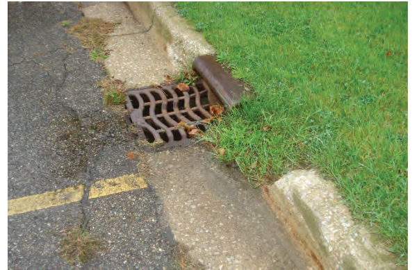
Photo 2: Broken section of concrete curb and gutter
