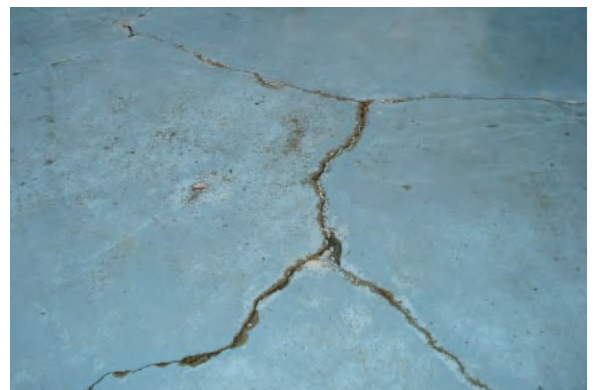
Photo 1: Concrete cracking and vertical displacement
