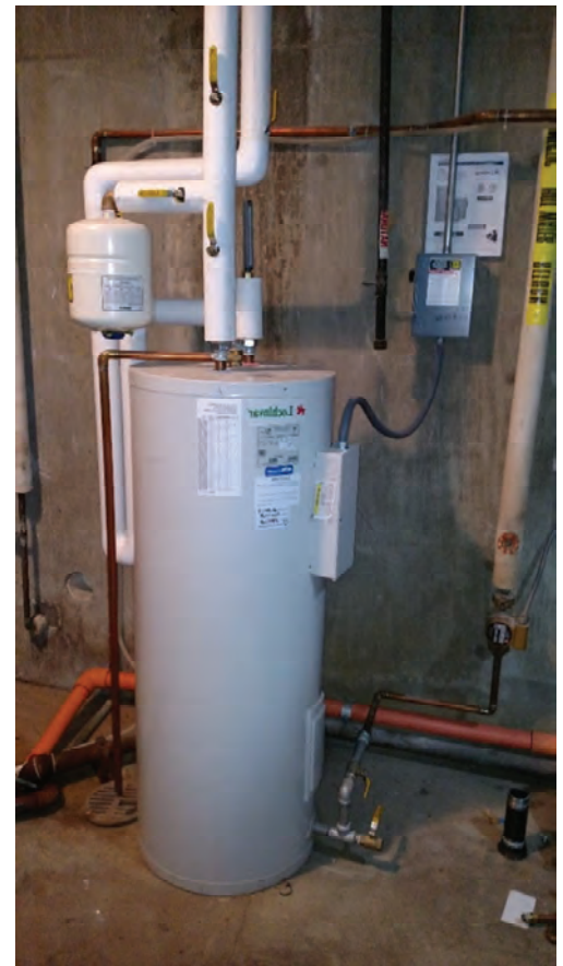
PLMB #4 Electric Water Heater
