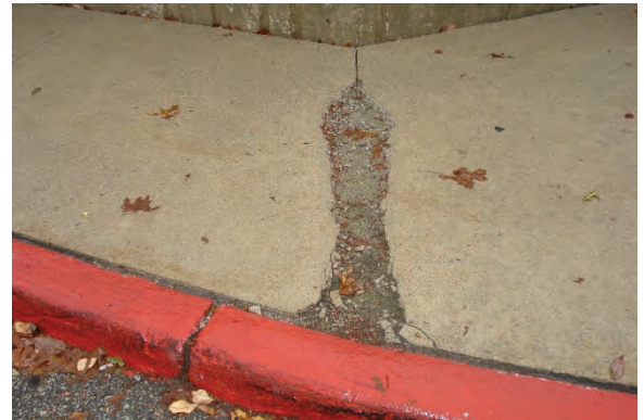
Photo 3: Deteriorated concrete sidewalk joint
