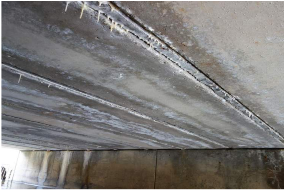
Typical Leaching Joint Between Box Beams
