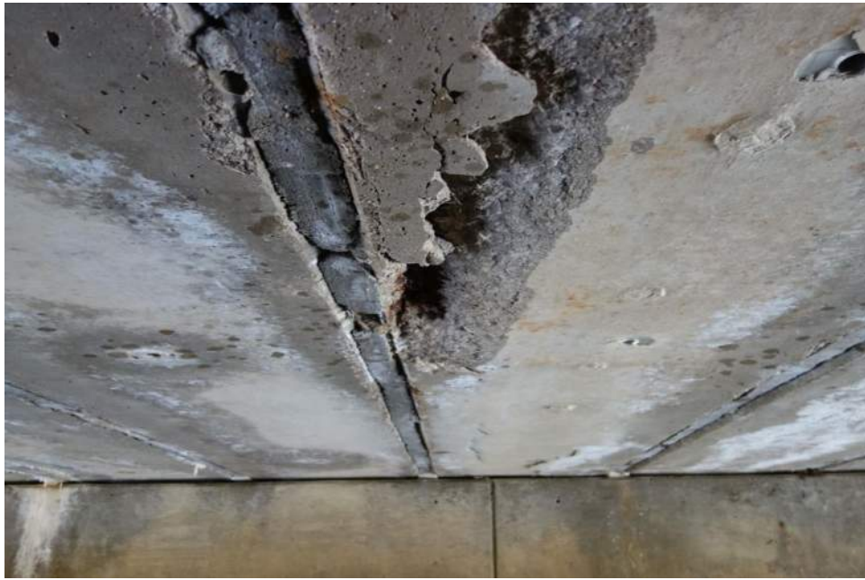
Beam 7W Delamination and Broken Strand
