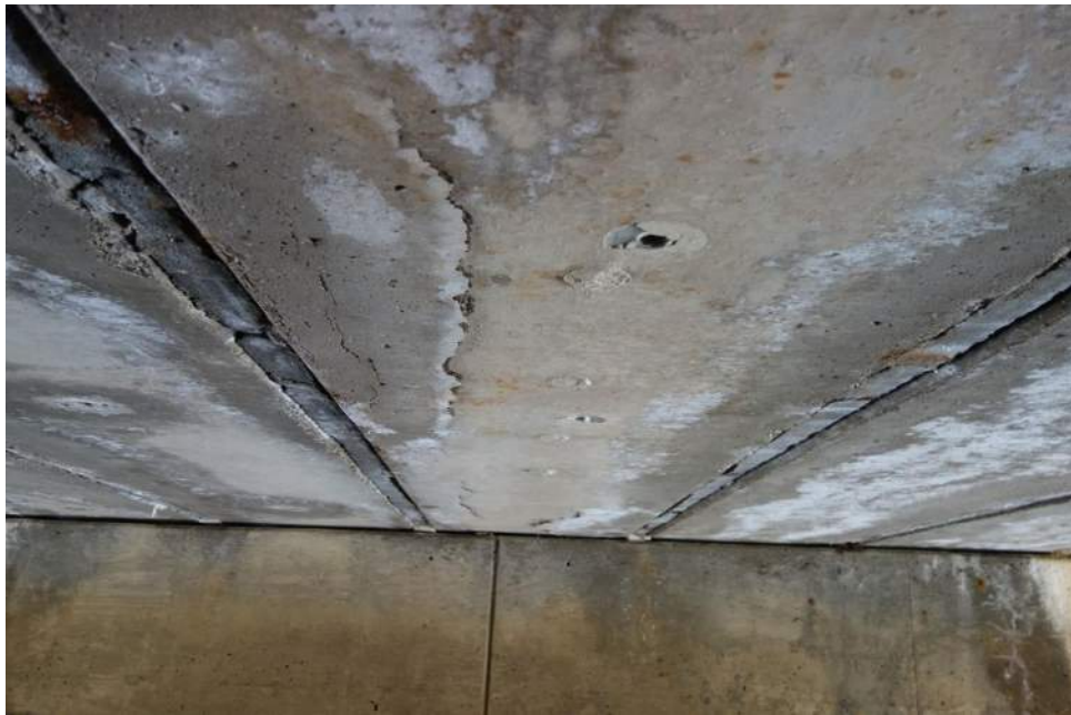
Beam 5W Cracking
