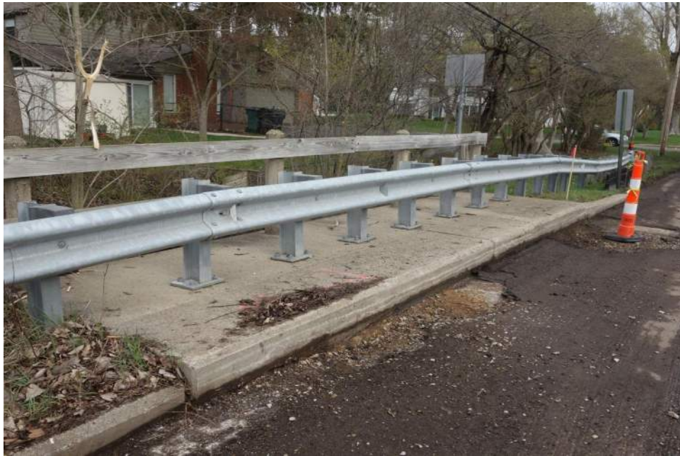
Top Flange of Box Beam Deterioration
