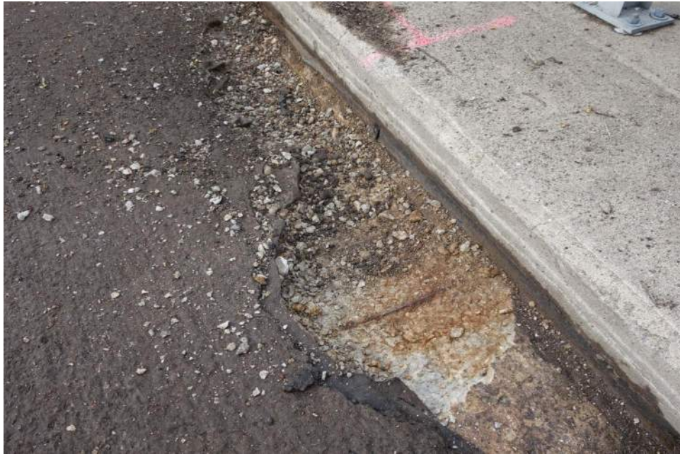
Top Flange of Box Beam Deterioration
