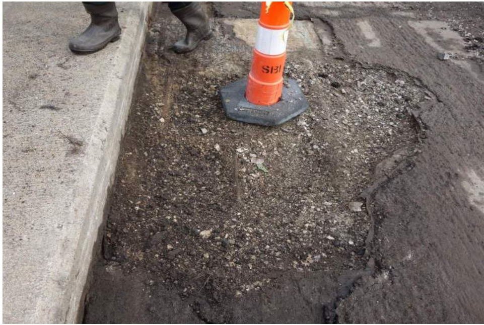
Top Flange of Box Beam Deterioration
