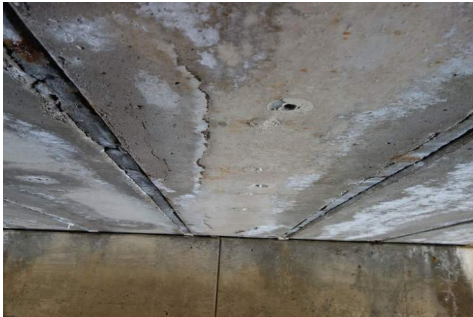
Beam 5W Cracking
