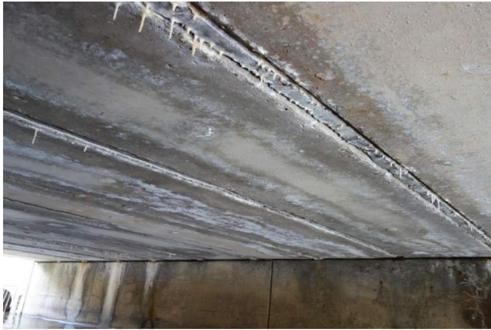
Typical Leaching Joint Between Box Beams
