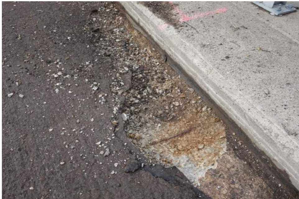
Top Flange of Box Beam Deterioration
