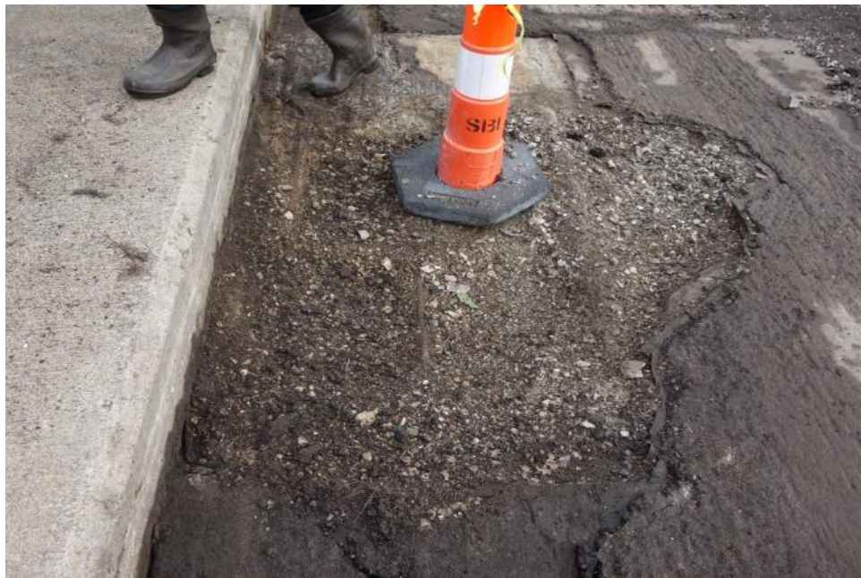
Top Flange of Box Beam Deterioration
